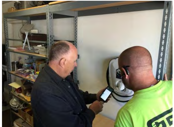
Residential EVSE installation with direct load management capability via homeowner WiFi and the Greenlots network (2017)
