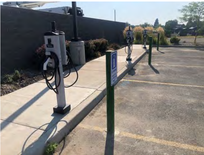
Workplace and Fleet EVSE installed for the City of Spokane (2019)
