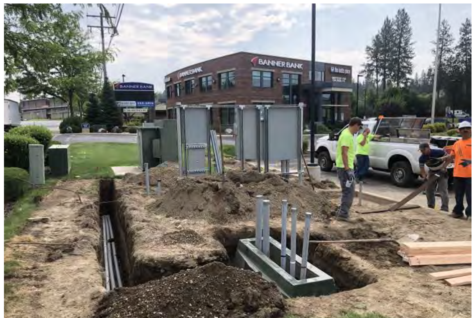
DCFC site under construction at Wandermere shopping center, in partnership with Washington Trust Bank (2018)
