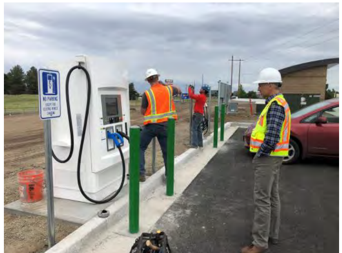
DCFC site construction at the West Plains Transit Center and Park & Ride—in partnership with Spokane Transit Authority (2018)
