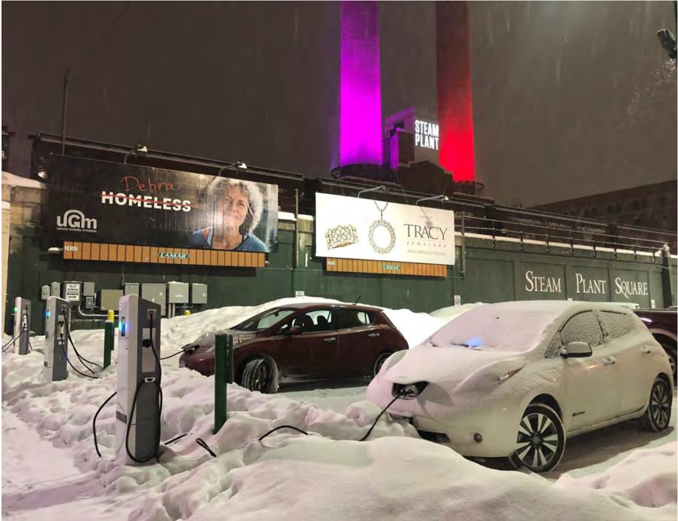
Public AC Level 2 EVSE at Steam Plant Square in downtown Spokane (2018)
