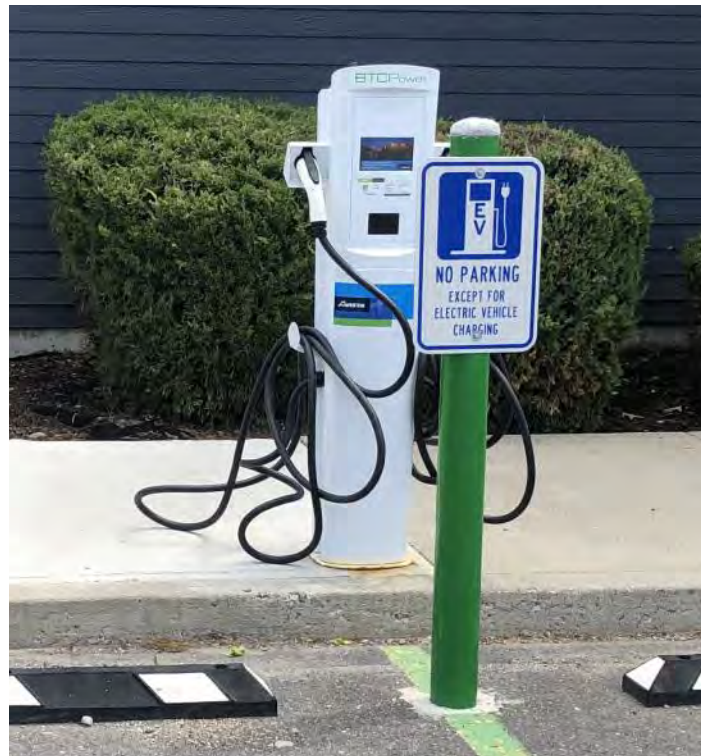
Avista EVSE for fleet, public, and workplace charging — Spokane Project Center (2017)
