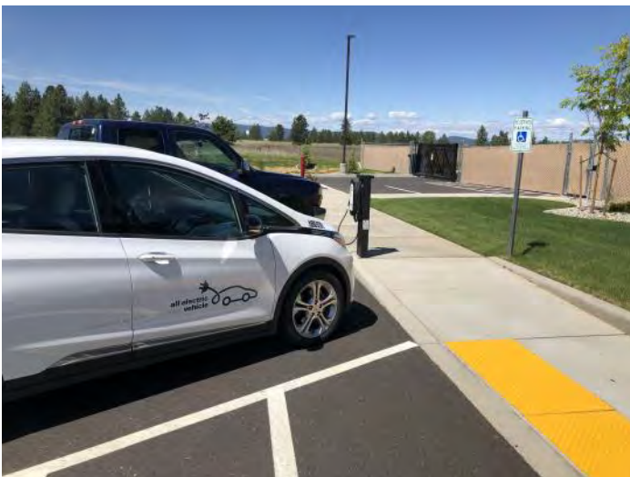
Avista fleet EV and facility EVSE for fleet, public, and workplace charging — Deer Park, Washington (2018)
